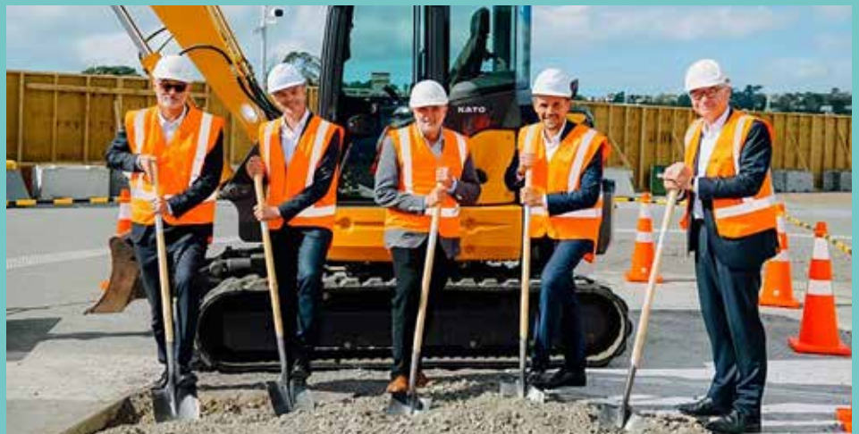
Dignitaries from Willis Bond, Architectus and Kainga Ora breaking ground at the Catalina Bay Apartments development in Hobsonville Point, Auckland.
