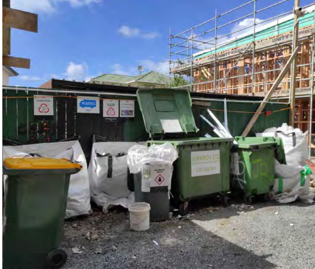
The construction industry is one of New Zealand’s biggest waste-to-landfill contributors, but pioneering construction “waste-warriors” are re-purposing huge amounts of waste into reusable building products.
