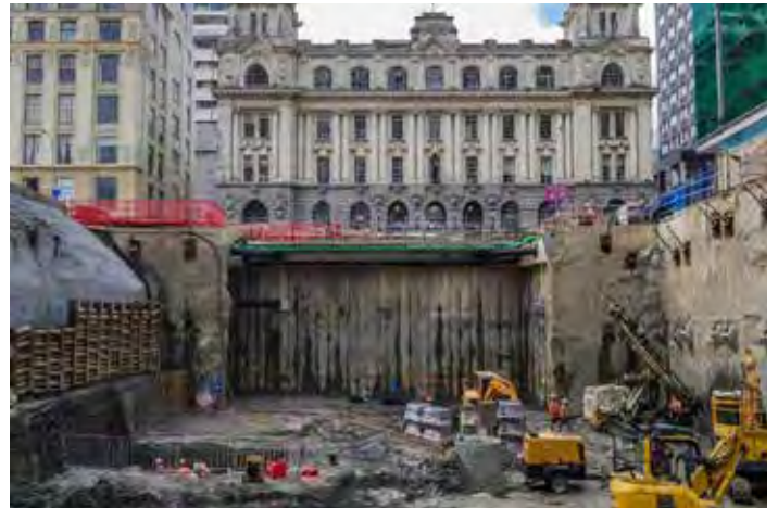
City Rail Link C1, Chief Post Office and Lower Queen Street, Auckland.
