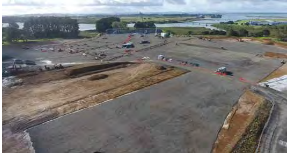
Major construction has started on Manawa Bay, Auckland Airport's $200 million-plus premium retail centre.
