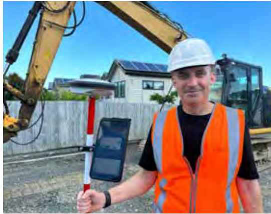
beforeUdig operations manager and utilities damage prevention expert Phil Cornforth with essential equipment for safe digging prep.
