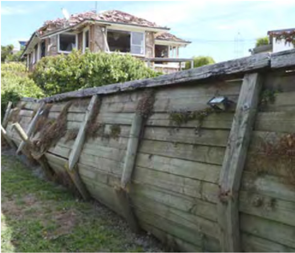
Damage to a retaining wall following the 2011 Christchurch earthquake.
